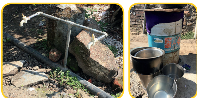
Community tap and water storage equipment in Ram Nagar, Pune
